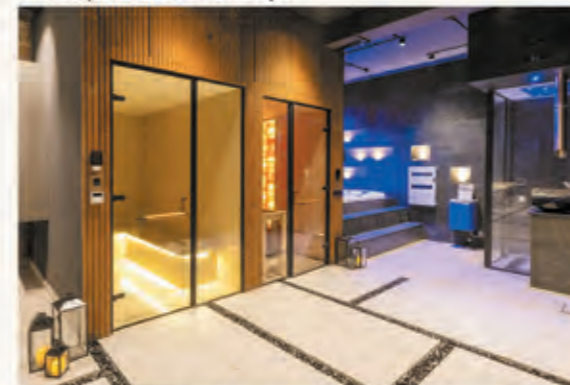
Spa Wet Area Equipments
